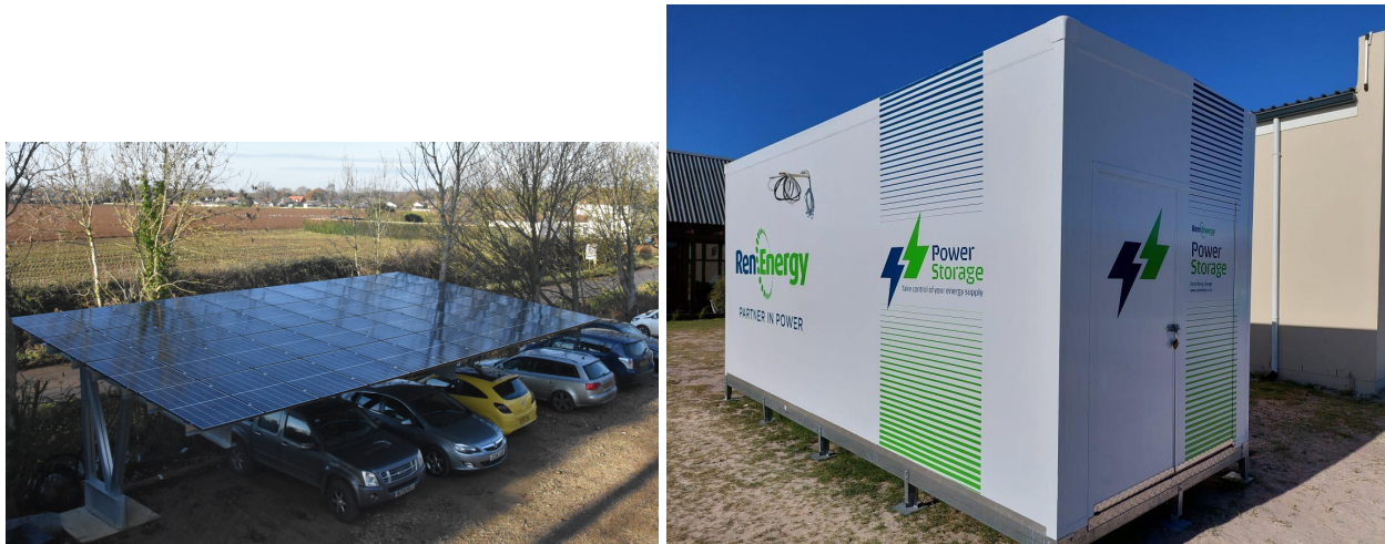
Figure A5.6: Solar canopy and static battery offering a renewable energy solution to ECP electricity supply.
